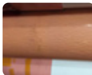
These small cracks are all running in the same general direction which tells us they were caused by high ozone levels in the air.
